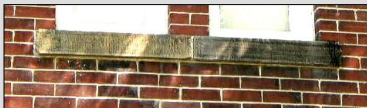
The plinth of the walls and the sills of the openings are made of cut limestone, obtained from the John Rogers Dry Goods Store on Queen Street, which was demolished c1900.
